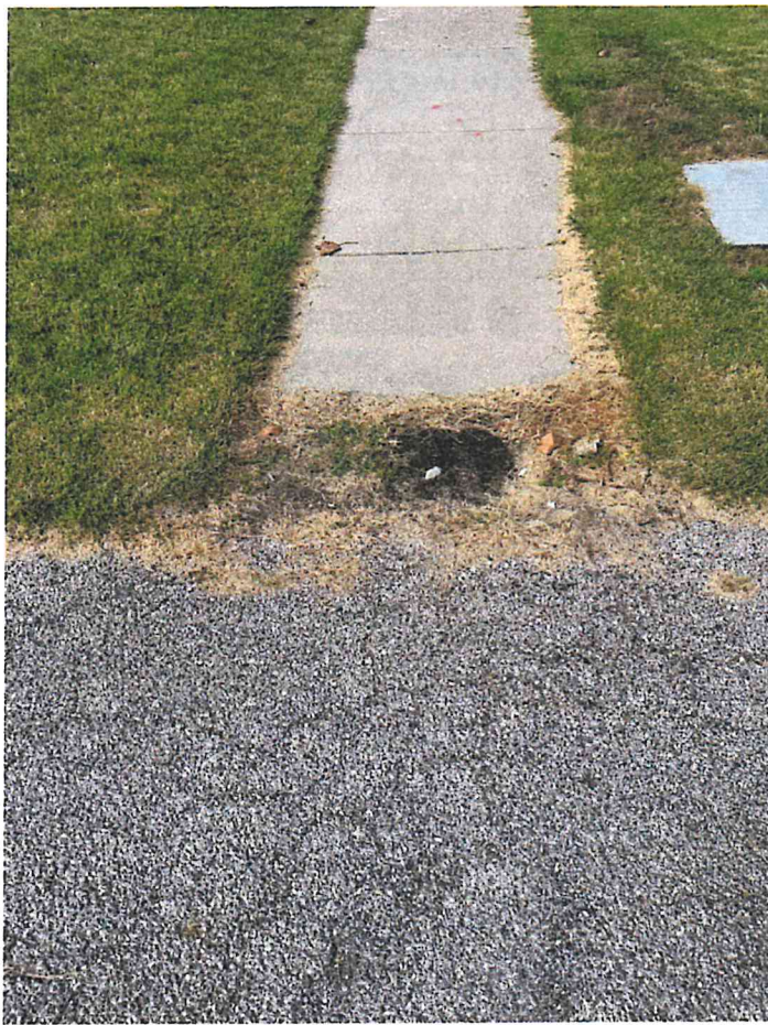
Bad section of sidewalk in front of 420 N. Klein St.
